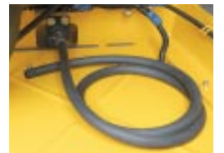
The engine oil drain valve was attached remotely, and connected the drain hose
