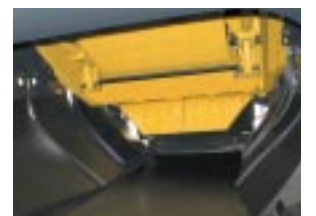
Between the crusher discharge and the belt conveyor
