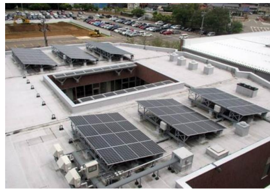
Examples of solar power generation (Awazu Plant Solar Panel)
