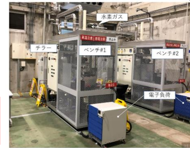
Fuel cell bench test facility
