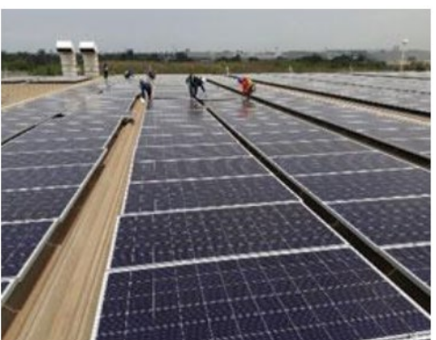
Solar panel introduced at Thai plant (2018)
