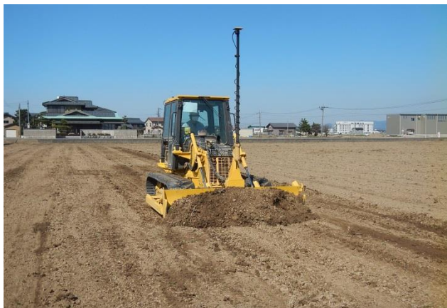
High-precision leveling of rice paddies by using multifunctional ICT-intensive dozer (Improved yield)
