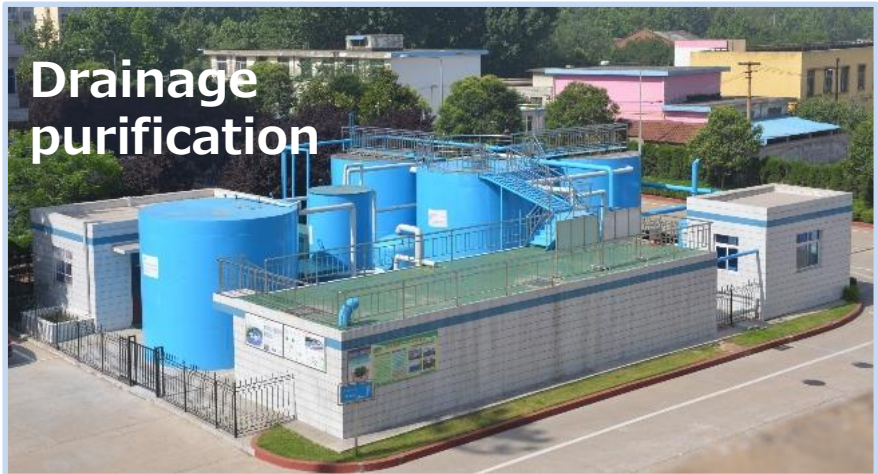
Chine (KSC) : Waste water treatment
