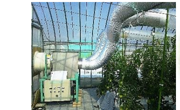
Groundwater-used cooling device Cooling inside the greenhouse in summer
