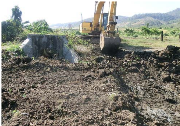
Discharged Hume pipe
