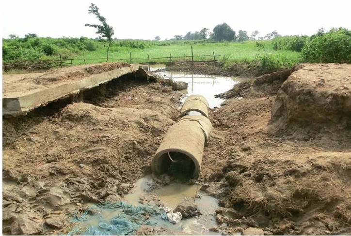
Road destroyed by floods
