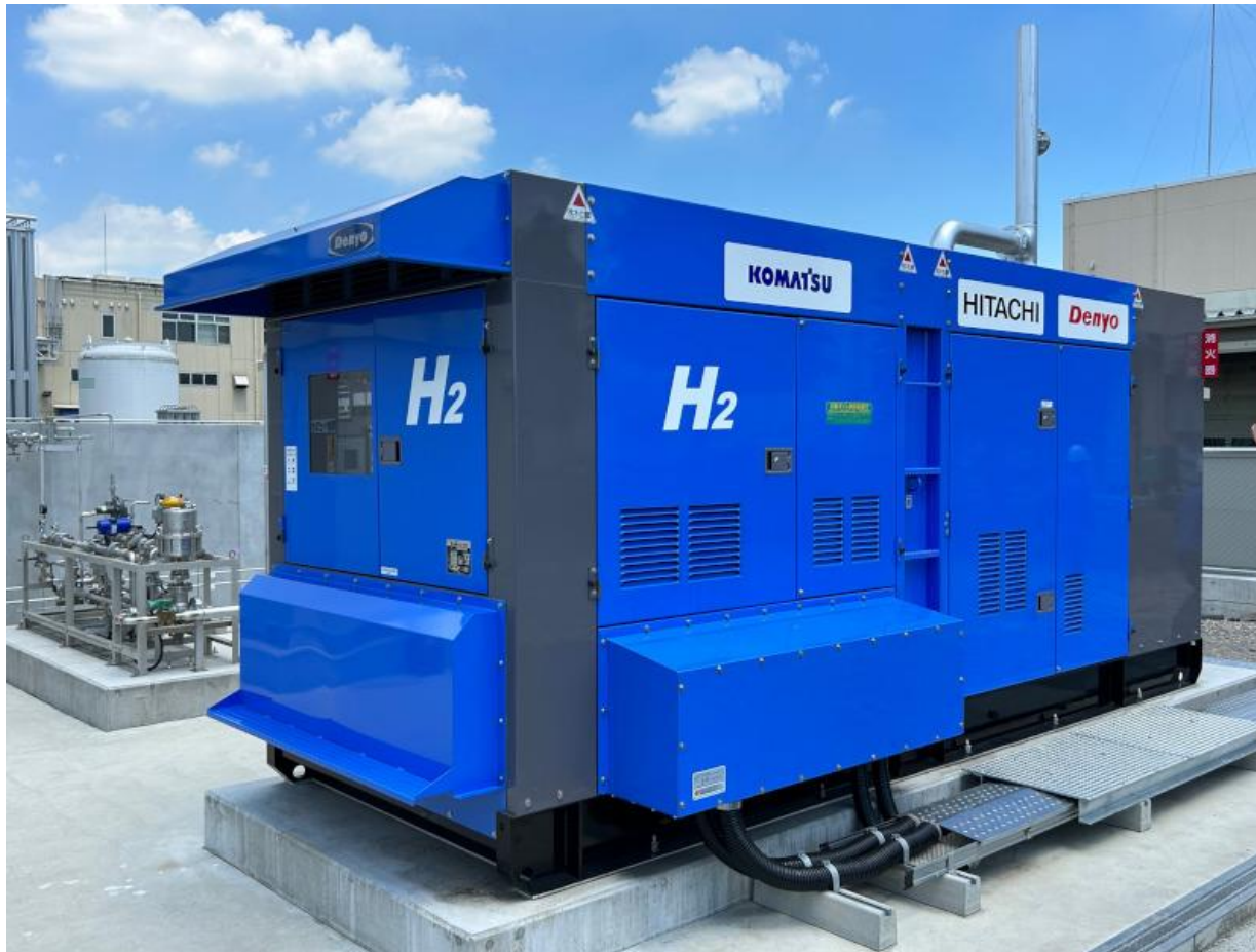
Hydrogen co-firing generator installed at Oyama Plant
