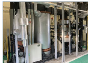
Biomass boiler at Ibaraki Plant
