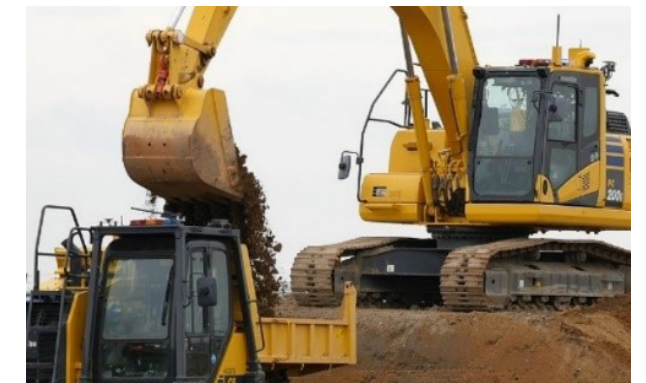
A demonstration showing a hydraulic excavator and a crawler dump truck, both completely unmanned, autonomously collaborating to excavate, convey via rotation, and load soil and then carry it to be expelled at a designated location.
