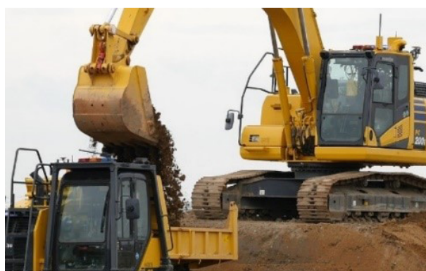
A demonstration showing a hydraulic excavator and a crawler dump truck, both completely unmanned, autonomously collaborating to excavate, convey via rotation, and load soil and then carry it to be expelled at a designated location.
